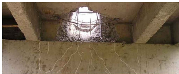
图 12 单跨面层、横梁出现贯穿性破坏 Fig. 12 Penetrating damage occurred in single span panel and cross-beam
