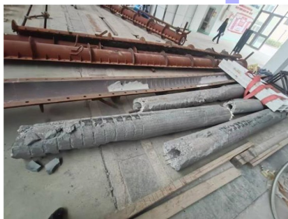
a) PHC 桩断裂
