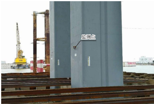
图 12 广深沿江高速桥墩竖向、水平位移监测点布置 Fig. 12 Layout of vertical and horizontal displacement monitoring points for piers of the Guangzhou-Shenzhen coastal expressway
