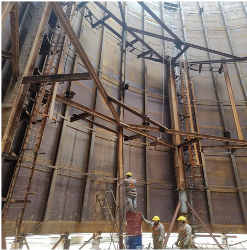
图 4 传感器的安装与保护 Fig. 4 Installation and protection of sensors
