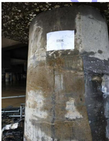
图2 码头桩基裂缝破损
